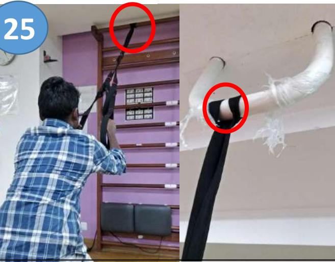
Fixation of hook to ceiling to prevent patient fall and damage to existing assets
